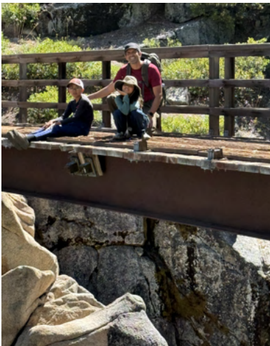
Damaged bridge over Highland Creek
